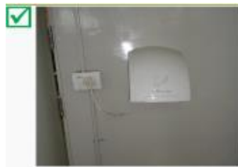
Fig 27 : Provision of hand dryer for drying hands at entrance
